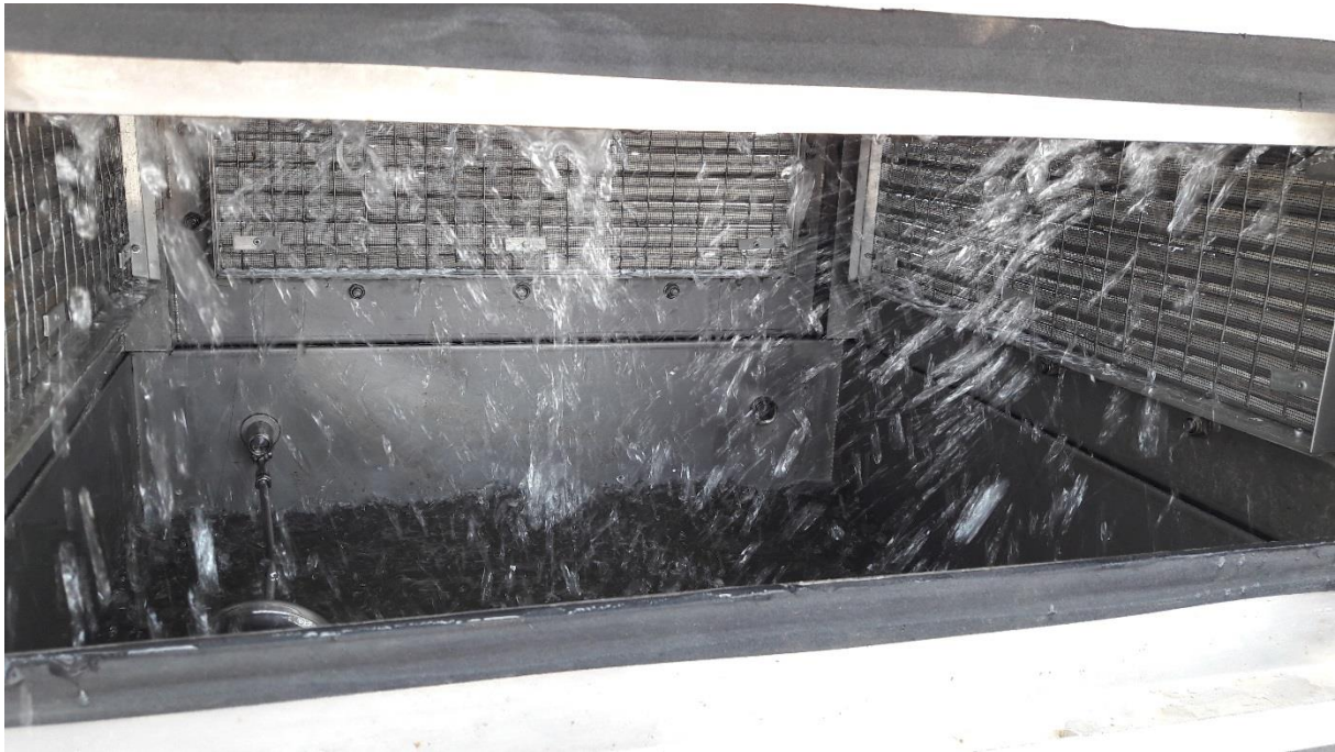
Figure 2.5: View of the sump during operation through the bottom hatch
